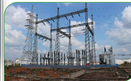
110MVA ELECTRIC POWER STATION 1 ST STAGE 30MVA
